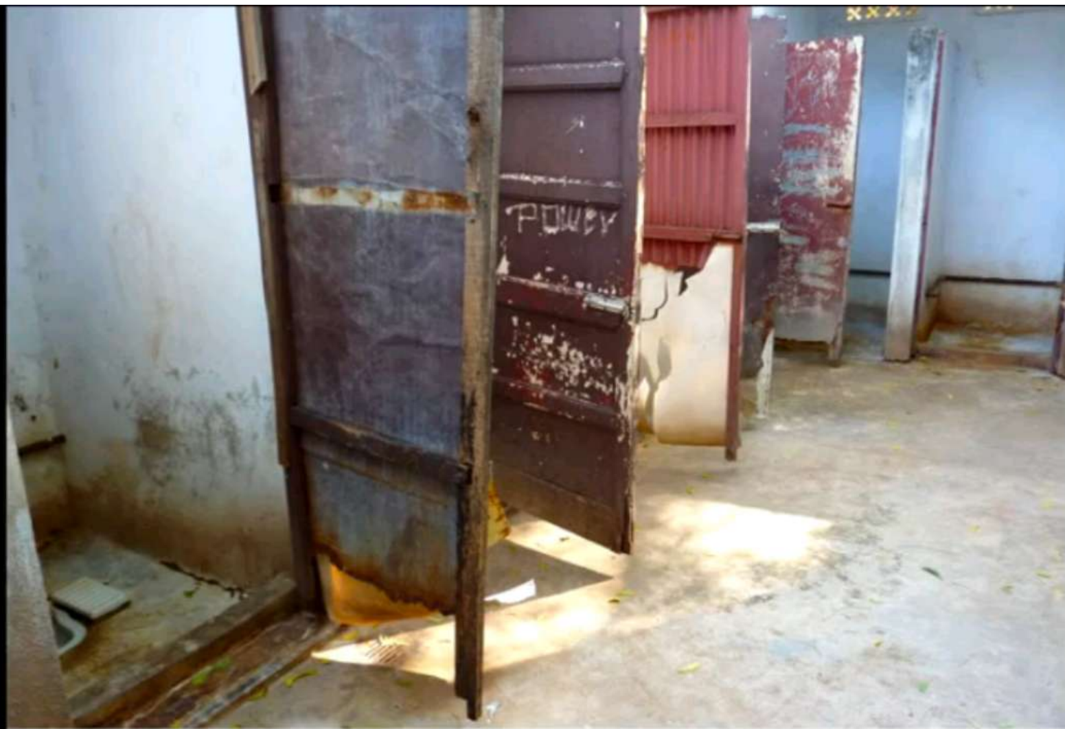
[BOYS TOILET]: Doors are barely usable. Pans are new, but note that toilets are tough to keep clean. This area being covered would be a benefit to their ability to effectively use the toilets.
