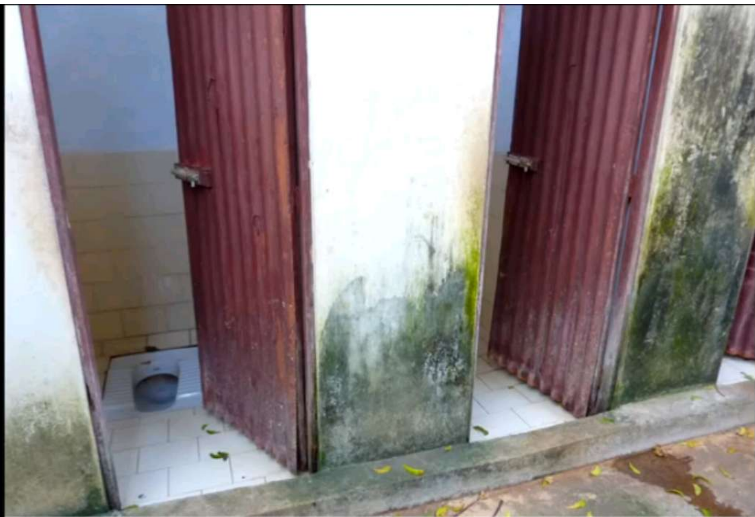
[GIRLS TOILET STALLS]: Shows renovations - new pans, AND new tiles provide great relief for ability to keep them clean. Doors are in better condition. There is no water supply into these stalls, which is still a problem.
