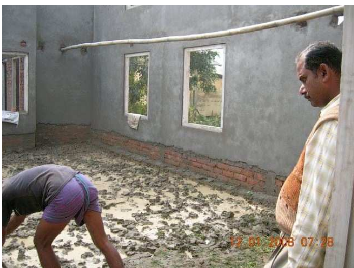
Work on Floor in Activity room (right in photo is sub contractor)
