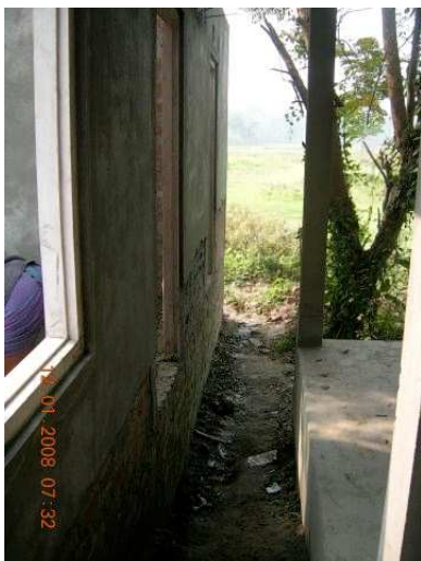
Left toilets and right class room. The area seen between is to be filled with sand to provide access to toilets.
