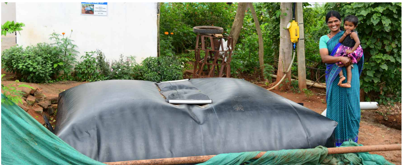
A Biogas Unit installed in front of Malliga's house
