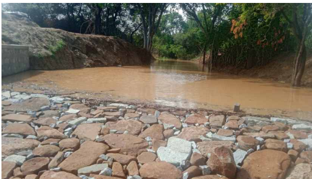
The check dam is holding the water and checking surface water runoff.
