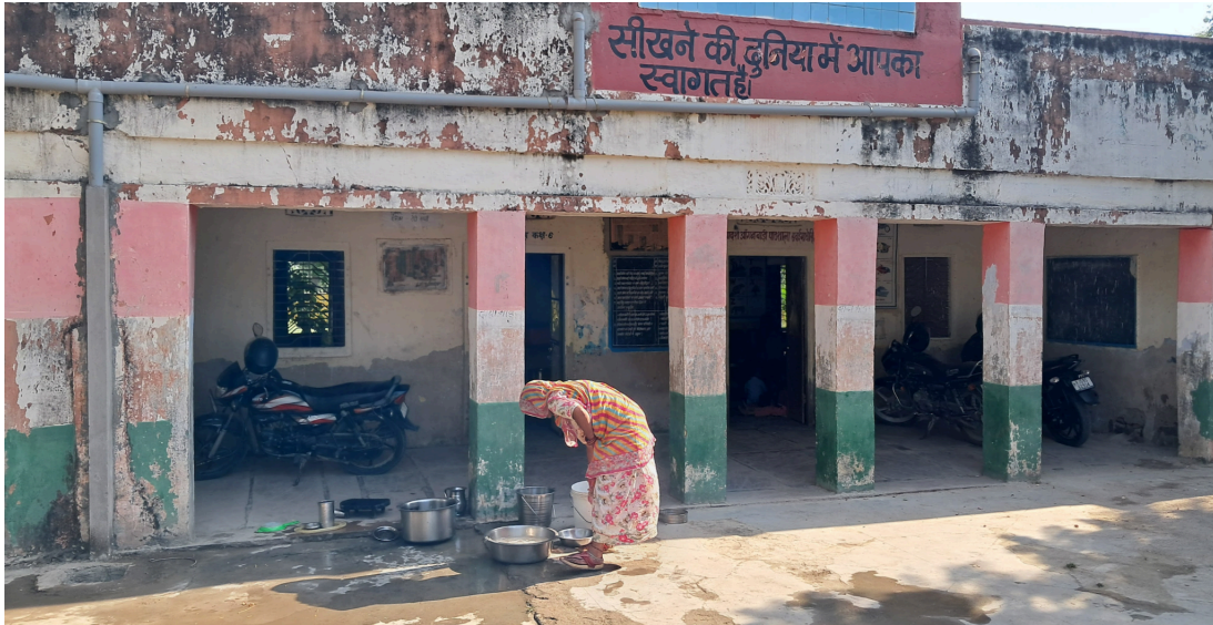
Pipes were connected to the existing terraces to redirect the rainwater in Jaipur
