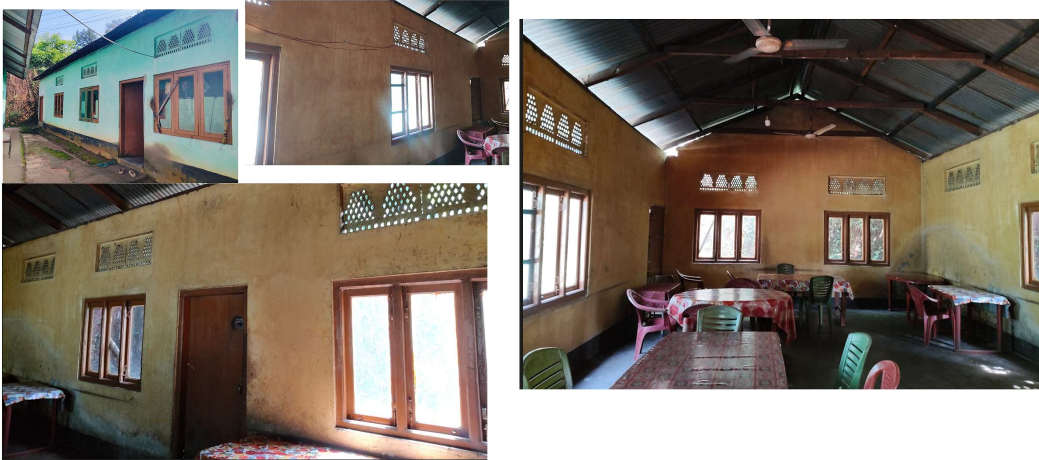
Kitchen & Dining Building: Stained interior and exterior walls with visible water-damage marks
